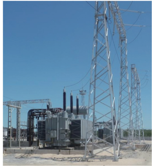
Electrical Substation at K&S
