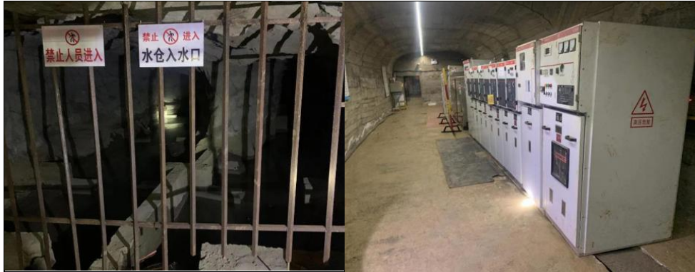
Figure 10-21: Photos of Main Sump and Power Substation on Adit Level of Dongfeng Mine
