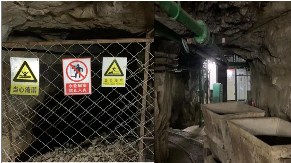
Figure 10-8: Photos of Level 5 Sump and Main Power Substation of Lianhuagou #5 Zone
