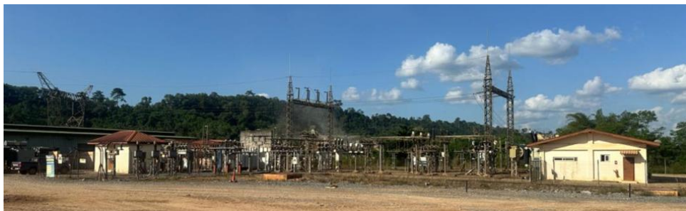
Figure 14-4: Main Transformer Station
