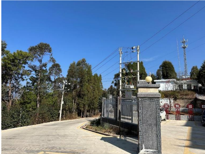
Figure 12-1: Power Station of Liantiexiang
