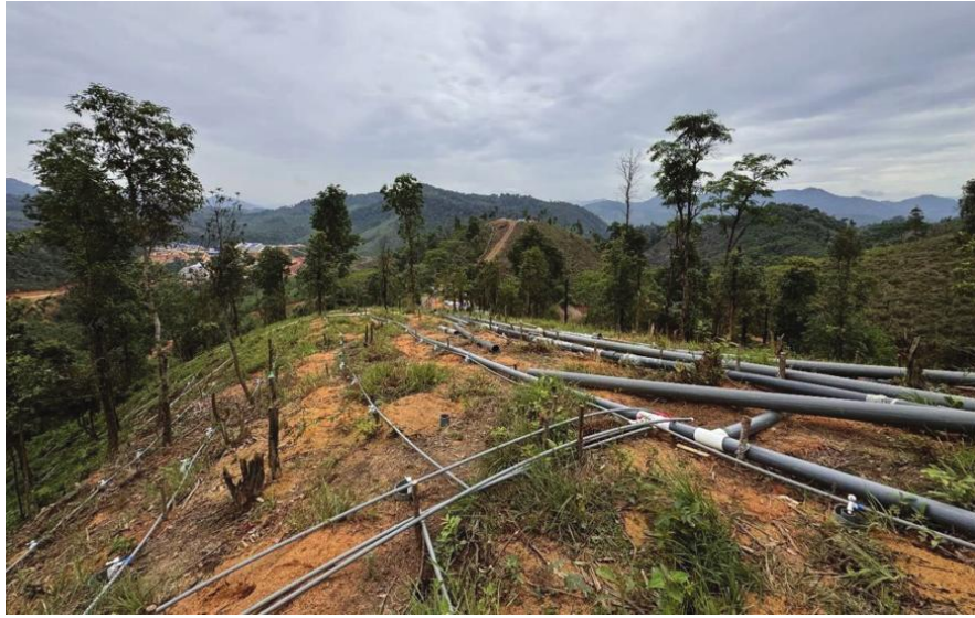
Figure 11-2: In-Situ Injection System at The Mountaintop
