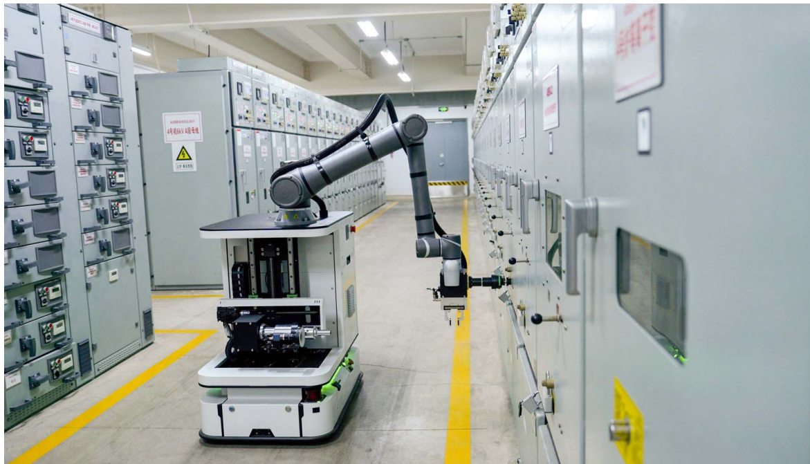
Conducting switching operation
