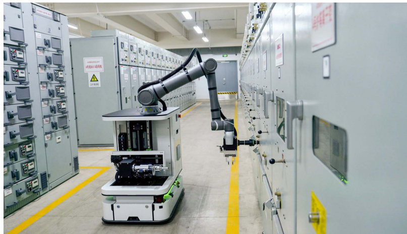
Conducting switching operation
