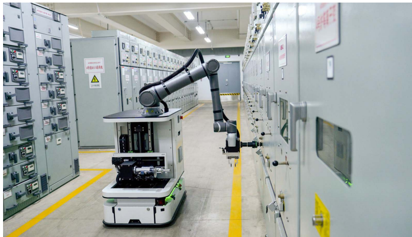
Conducting switching operation
