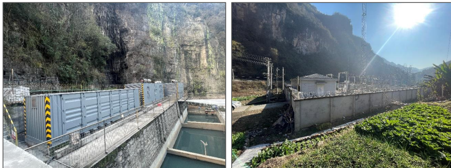
Figure 14-2: The Yanchi Substation (right) and Diesel Generator (left) Powering the Yulinxi Phosphate Mine
