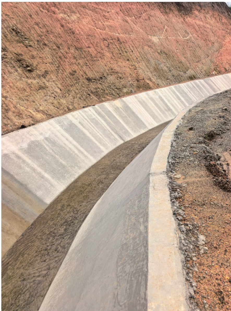
Figure 18.10: As-Built Containment Structures Downstream of the TSF and
