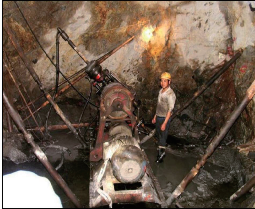
Figure 10.3: Underground Drill Rig XY-4
