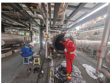
Performing eddy current testing on heat exchangers at the process station
