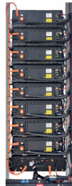
RelyEZ Liquid-Cooled Rack
