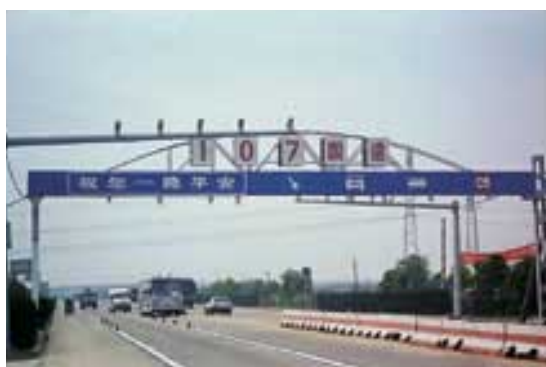
Recording equipment located in City Highway
