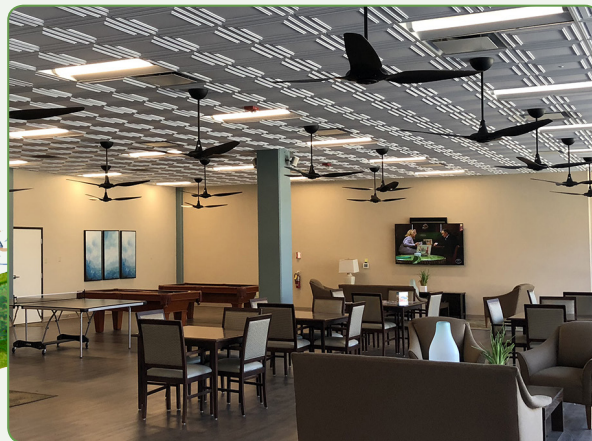
Figure 2. Ceiling Fans 圖2. 吊扇
