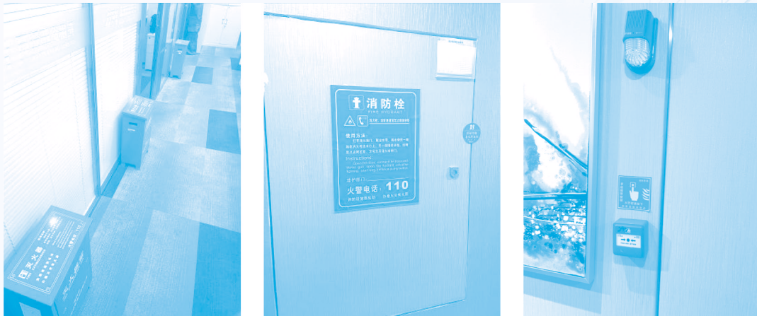
Fire safety equipment in the workplace 於工作場所的消防安全設備
