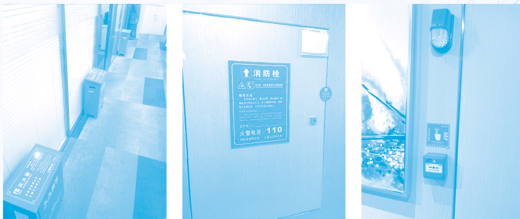
Fire safety equipment in the workplace 於工作場所的消防安全設備
