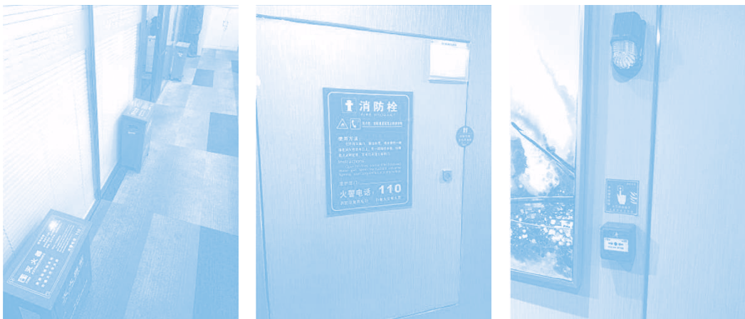
Fire safety equipment in the workplace
