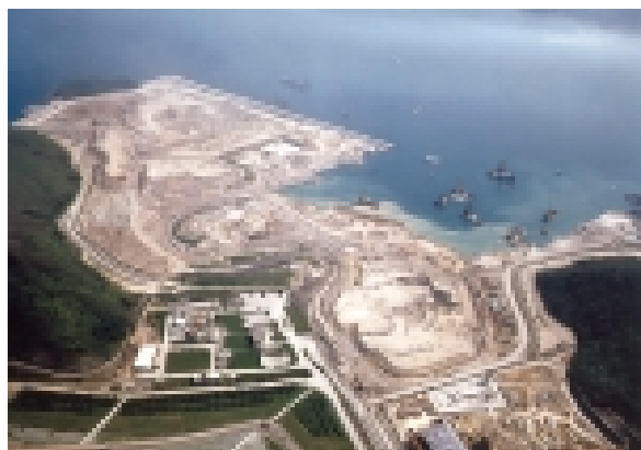
Construction of Seawalls and Reclamation at Tseung Kwan O Port Development at Area 137, Stage 2
