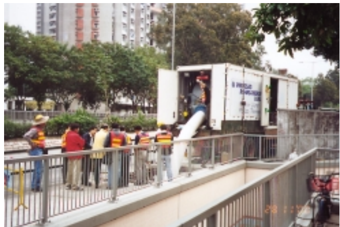
Relining of Asbestos Cement Fresh Watermain by Process Phoenix Structural Liner at Jockey Club Road
