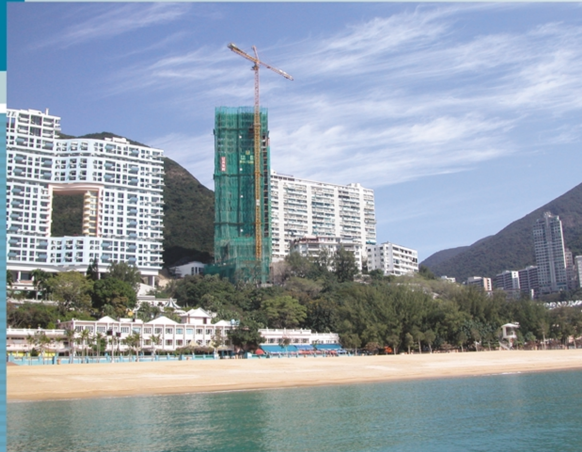
Luxurious residential development at Repulse Bay 淺水灣之豪華住宅發展項目
