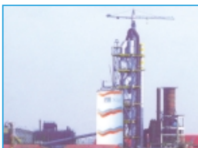
在建設中位於山東的聯合王晁廠房 Factory buildings of Allied Wangchao in Shandong under construction
