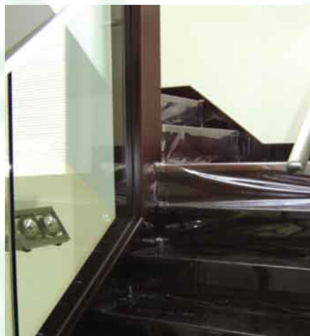
► Supply and installation of Polyboard and timber flooring for Le Bleu at Tung Chung 為位於東涌之水藍天供應及安裝百利板及木地板
