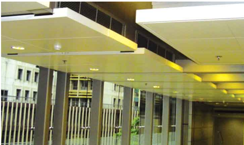
◀ Supply and installation of false ceiling for Police Headquarters at Wanchai 為位於灣仔警察總部 供應及安裝假天花
