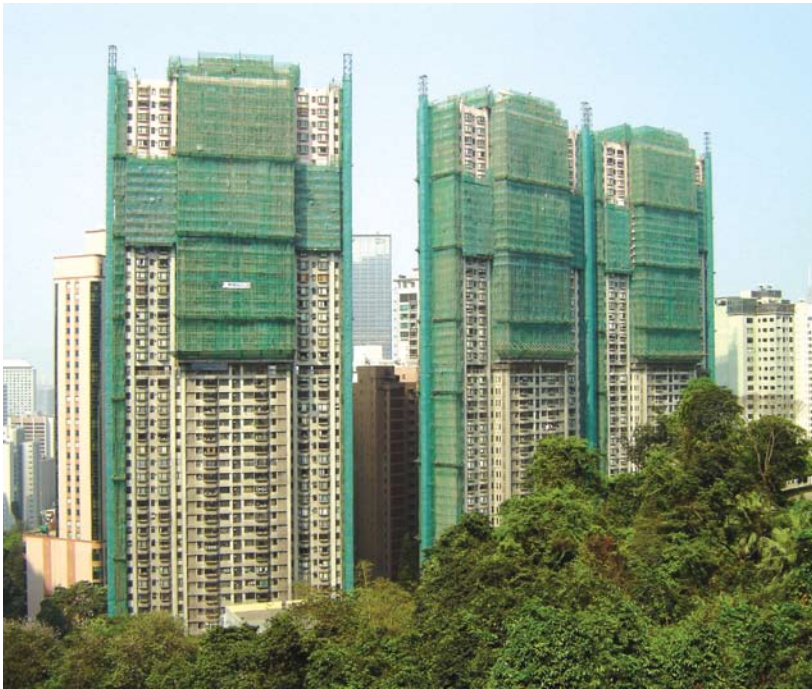
◀ Renovation works for Estoril Court at Garden Road 花園道愛都大廈維修工程
