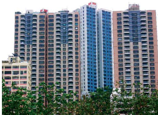
▲ External wall renovation works for Ventris Place in Happy Valley 跑馬地雲地利台之外牆維修工程
