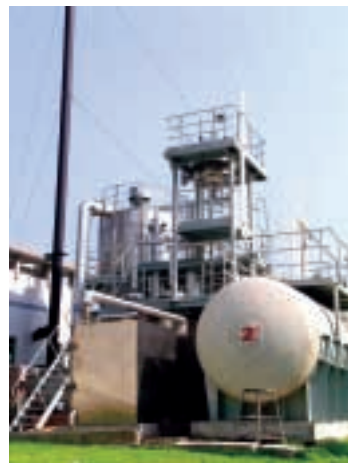
Heavy Water Treatment System
