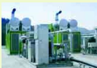
沼氣發電廠 Methane-to-energy plant
