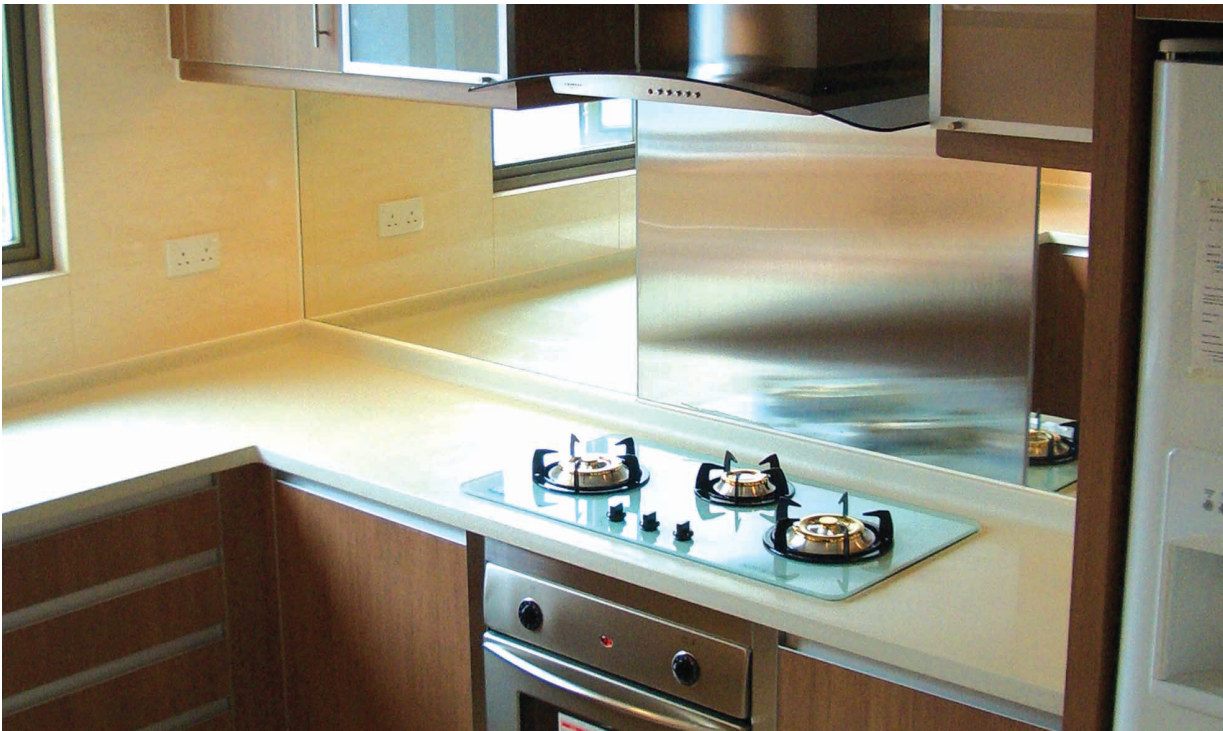
▲ Supply & installation of kitchen cabinets for The Portofino at Clear Water Bay 為清水灣栢濤灣供應及安裝廚櫃
