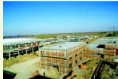
Zibo Hanmiao Waste Water Treatment Plant (under construction) 淄博韓廟污水處理廠（在建中）
