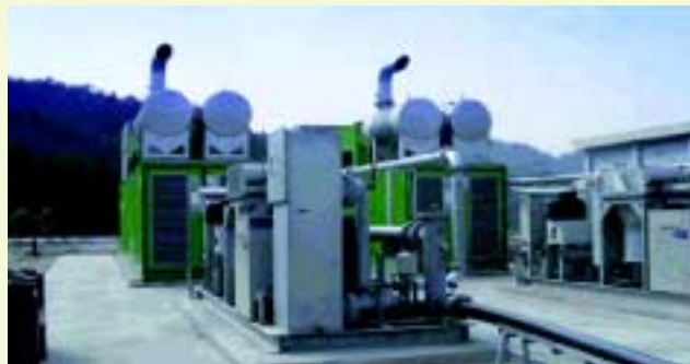
Methane-to-energy Plant 沼氣發電廠
