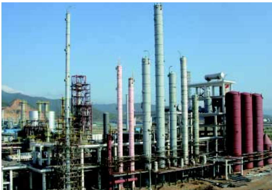
The phenol/acetone plant in Huizhou, Guangdong province further enhances our vertical integration development. 位於廣東省惠州之苯酚及丙酮廠，進一步提升集團之垂直整合發展。
