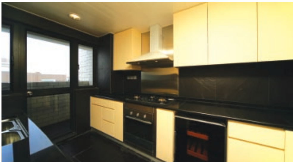
Supply and installation of kitchen cabinets for Kingsville Phase 2 in Macau 為澳門雍景灣第二期供應及安裝廚櫃
