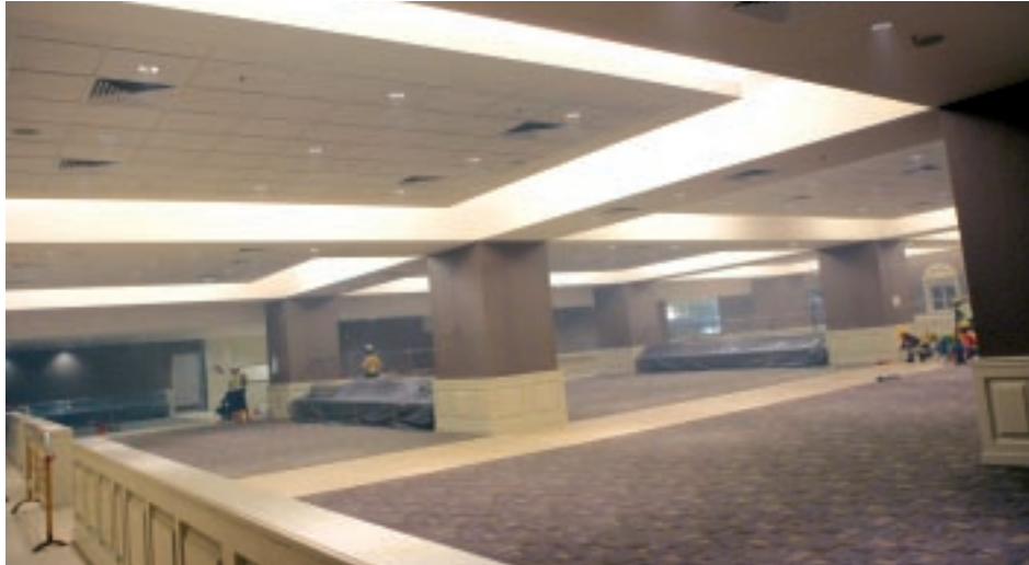
Supply and installation of false ceiling at Venetian Hotel Resort Development in Macau 為澳門威尼斯人渡假村酒店項目 供應及安裝假天花
