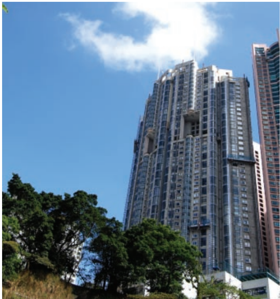
▶ Repairing and renovation work for Queen's Garden 裕景花園之修理及維修工程
