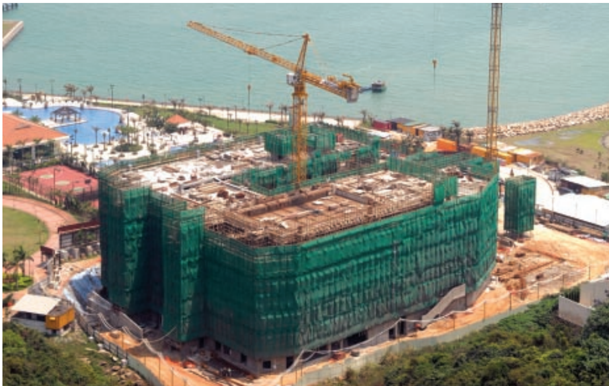
▲ Construction of a primary cum secondary school for the English Schools Foundation in Discovery Bay 為英基學校協會於愉景灣興建中小學
