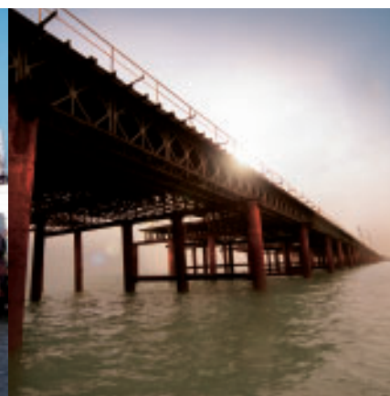
Yellow Sea Crossing-linking the man-made island and industrial and logistics park 連接人工島及工業物流園的黃海大橋
