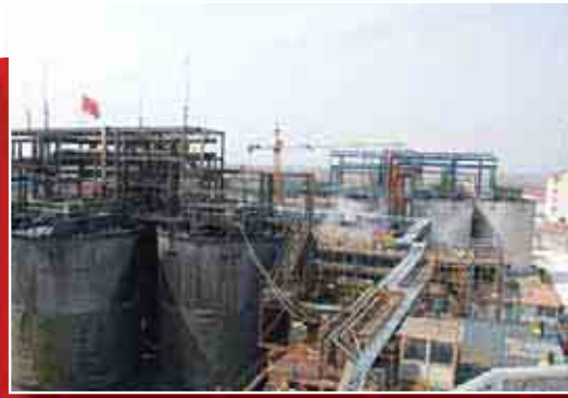
BioGold BACOX® processing tanks
