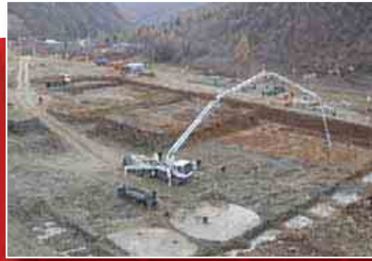
White Mountain plant site in October 2007
