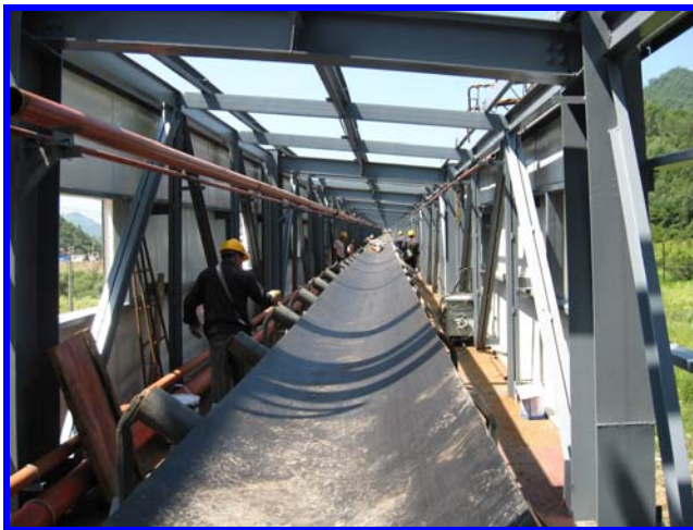
Ore conveyor belt installed
