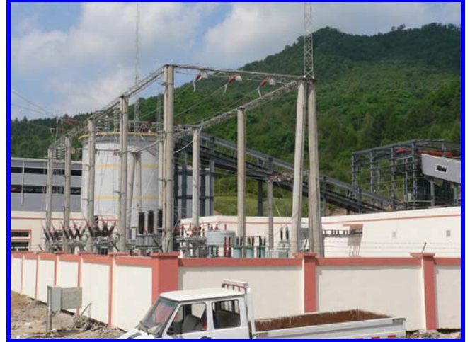
Electrical sub-station (now connected to mains power supply)
