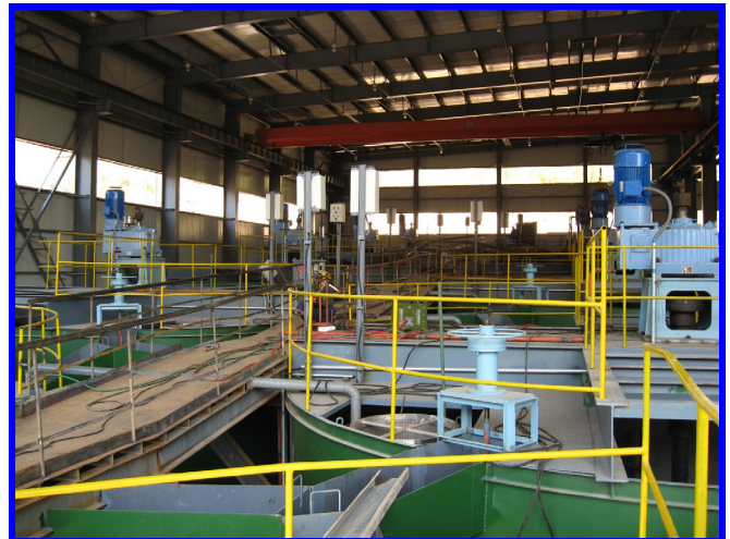
Commissioning of CIL tanks
