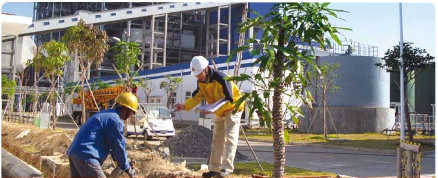
Fangchenggang supercritical plant in Guangxi, China
