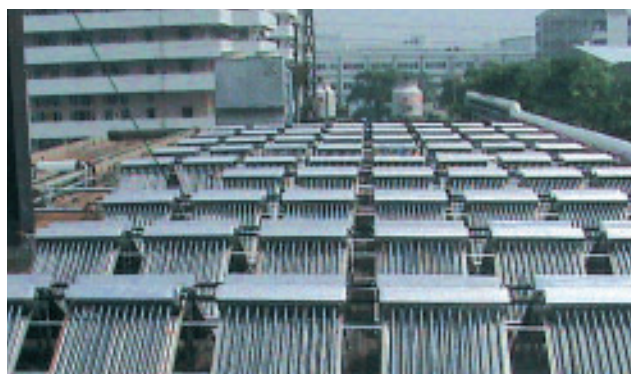
Solar panels at the Prime Asia Leather factory facility enabling natural sunlight to heat the water added in the leather manufacturing process. (Huangjiang Dongguan) 東莞黃江的普愛亞細亞皮革廠房設施的太陽能板，有助利用自然太陽光加熱皮革製造過程中所注入的水。
