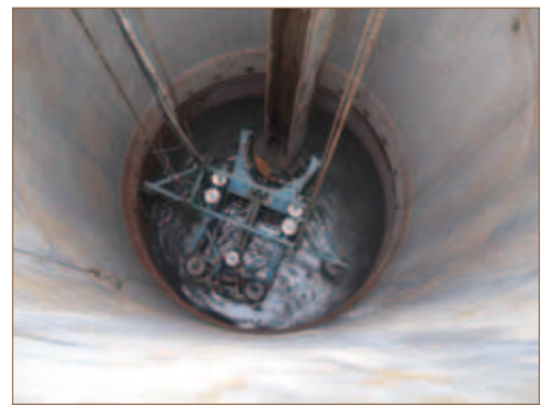
3. Robotic Cutting Method - Sink robotic cutting machine and cut H-pile 機械切割法 - 將機械切割機垂下及切割工字樁
