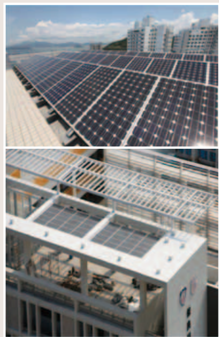
PV Panels at Li Shu Fan Building, HKU and So Kwun Wat Primary School 香港大學李樹芬樓及掃管笏小學之太陽能面板
