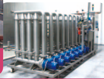
Cross-flow filter installed in Yantai Winery 煙台工廠錯流過濾機
