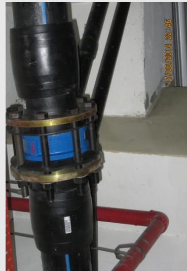
New Flood Mitigation Pump
