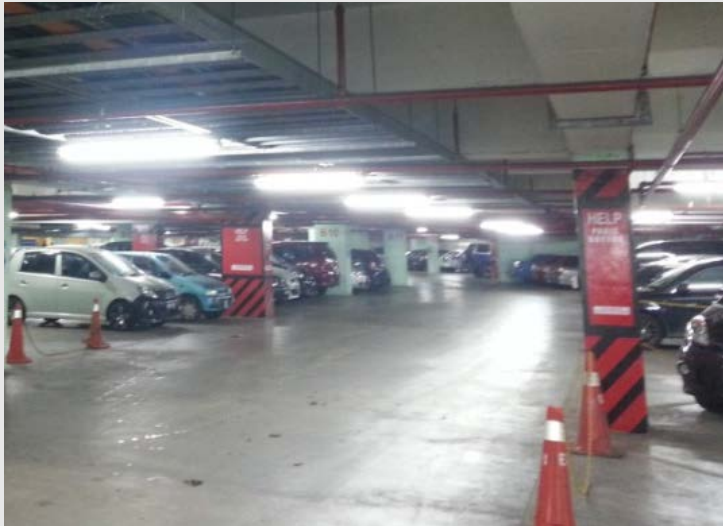
New T5 Lighting at Basement Car Park
