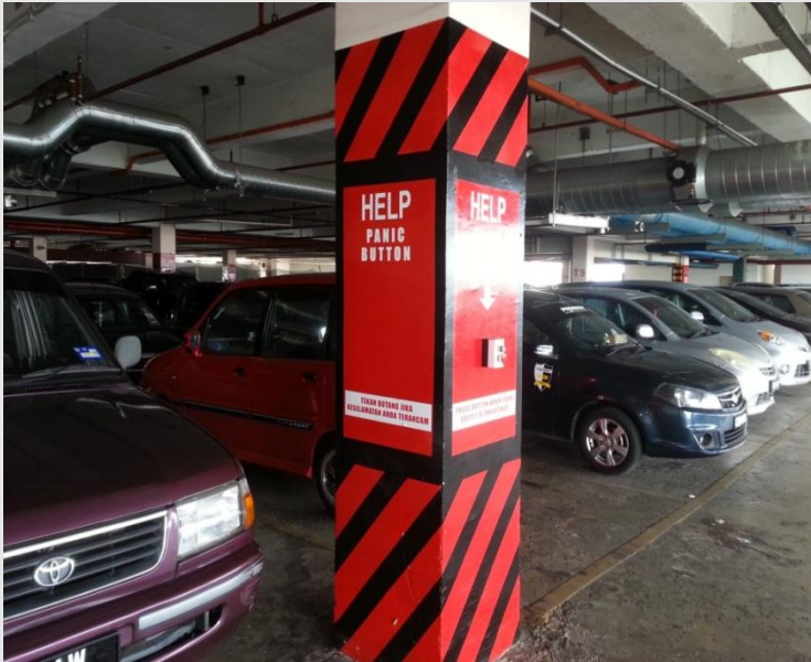
Panic Button Installed at Basement and Level 3 Car Park
