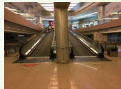
華潤五彩城電梯變頻改造項目 Variable-frequency escalator upgrades in Beijing Hi5
