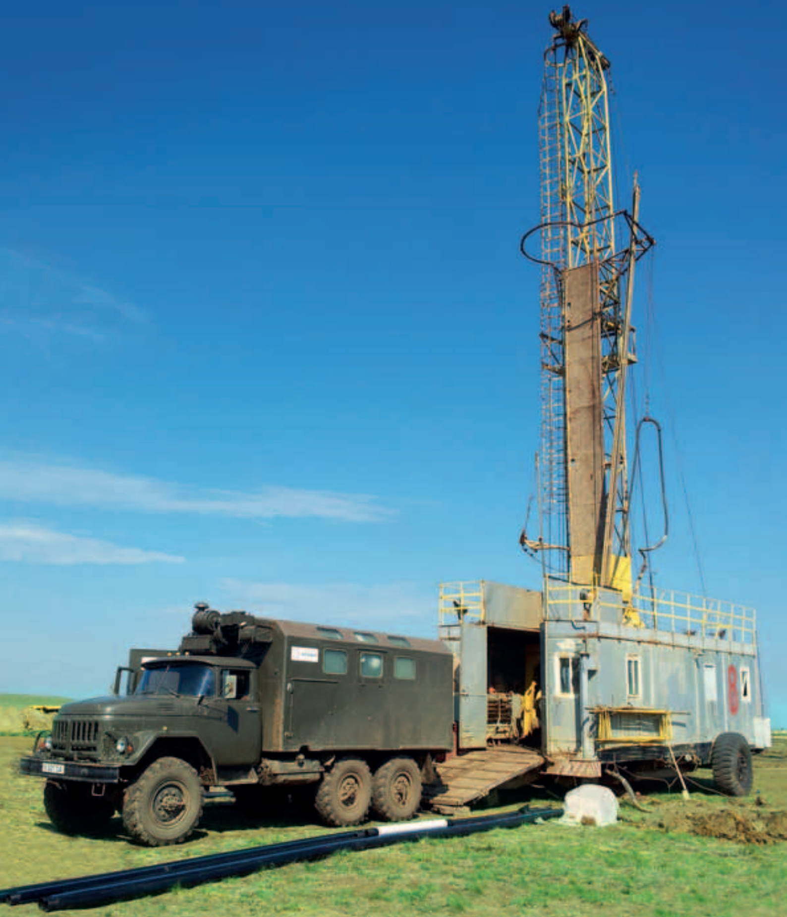
Drilling activities on the site of Semizbay-U 謝公司井場鑽孔施工場景
