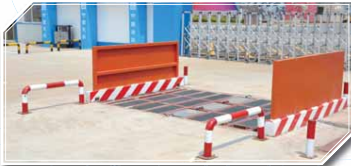
Car-washing trough at the entrance 出入口洗車槽
