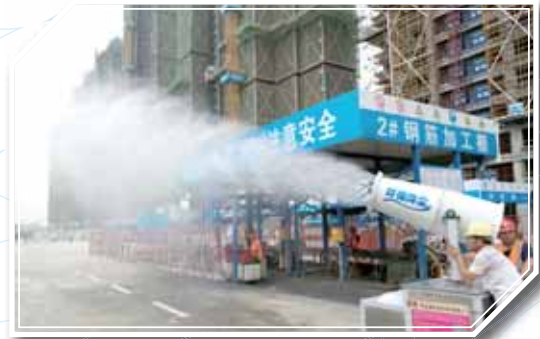
Water sprays to prevent dust at construction site 施工現場霧化降塵
