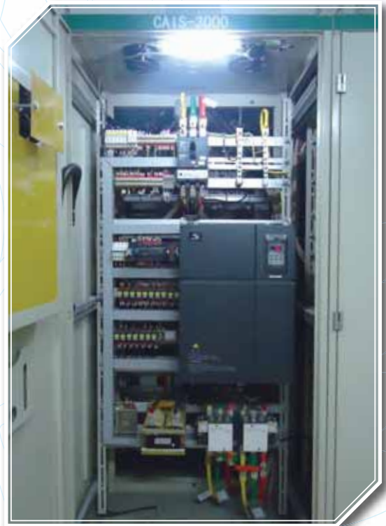
Variable-frequency controller for cooling pumps 冷卻泵變頻控制器
