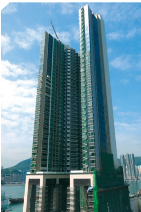
Proposed residential and commercial development at No. 5 Tung Yuen Street, Yau Tong, Kowloon 九龍油塘東源街5號建議住宅及商業發展項目
