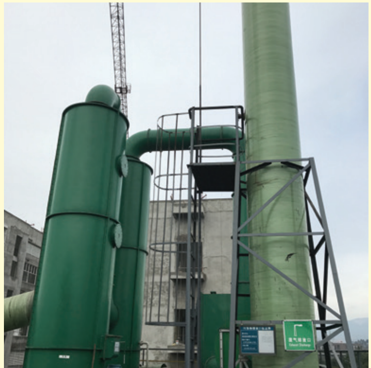
重慶康樂製藥有限公司處理廢棄物設施 — 車間廢氣治理設施 Waste disposal facility of Chongqing Kangle Pharmaceutical Ltd. — Waste gas treatment facility
