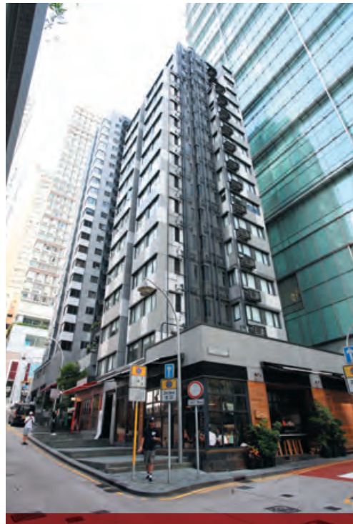
Refurbishment works for Regal Court and Wing Fung Building 永豪閣及永峰大廈之翻新工程
