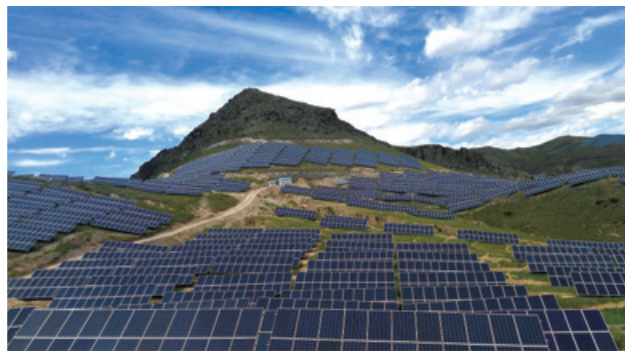
Hebei Yu County Photovoltaic Power Plant Project – BECE's first self-developed photovoltaic power plant
