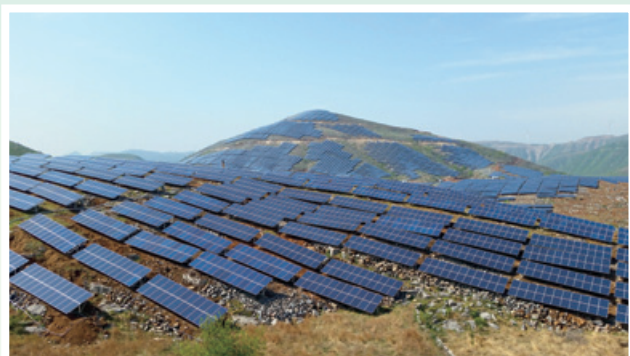
Qi County Miaokou Baisi Village Hillside Photovoltaic Power Plant Project 淇縣廟口鎮白寺村荒山光伏發電站項目
