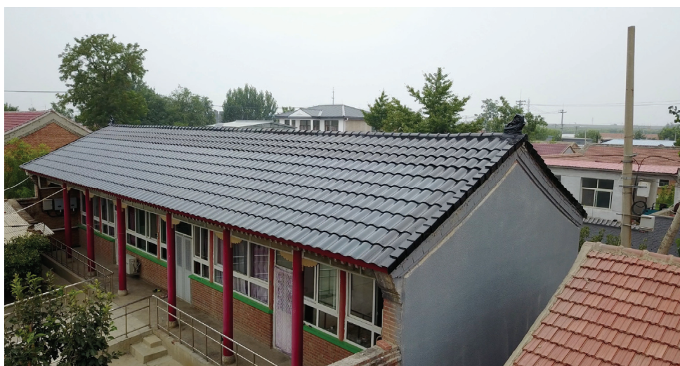
The Application of Hantile on the Roof of a Customer's House in Shunyi District, Beijing
