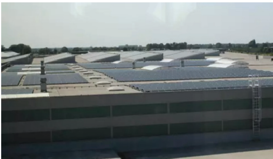
Rooftop Thin Film Power Generation Project at Plantion, a Plant and Flower Auction House in the Netherlands
