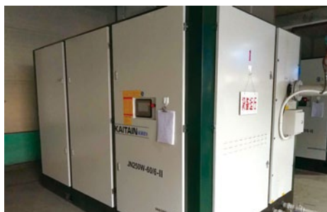
Shangdong Lanyan Air Compressor System Transformation 山東蘭雁空壓機系統改造
