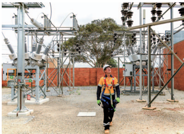
United Energy deploys advanced network infrastructure.
