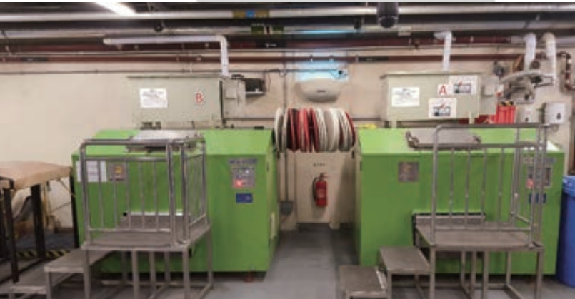
Biodegradable food waste decomposers are installed at City of Dreams to convert food wastage into organic fertilizer.
