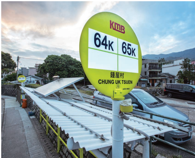
KMB has installed solar panels on the rooftops of bus shelters without an electricity supply 九巴為沒有電力供應的巴士候車亭安裝太陽能供電裝置
